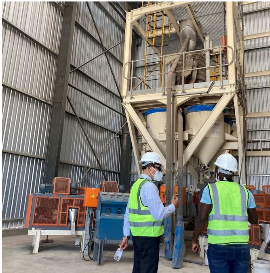
Ambassador Nishimaki (left) viewing the wet high-intensity magnetic separation (WHIMS) modules.
