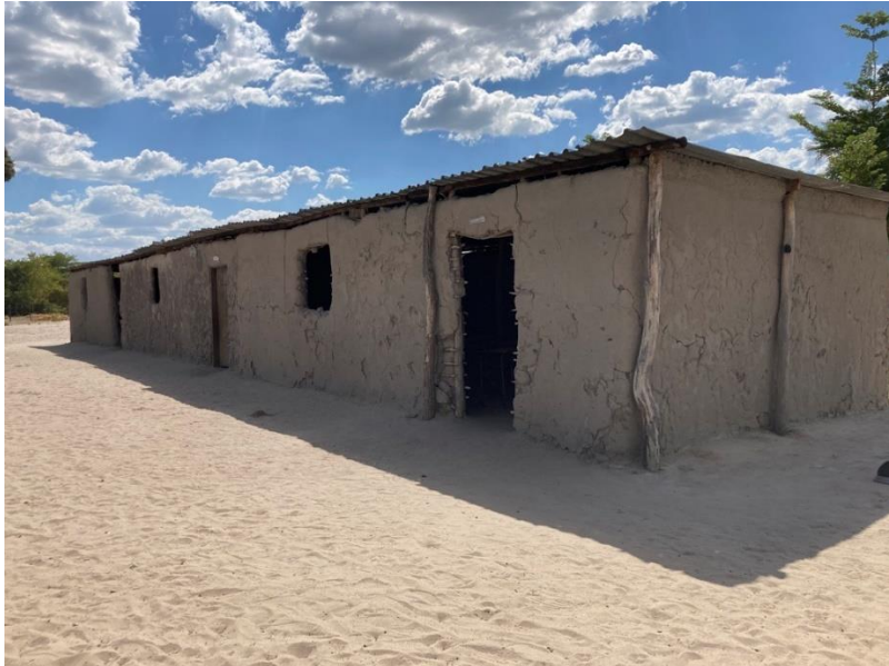
Photo 3: current classroom block (if it rains, there is a risk of the walls collapsing and water into the leaking electric circuit)
